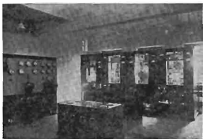
This modern ten-kilowatt transmitter of "Radio Maroc" may be heard on 23.3 and 37.3 meters. It is located at Kabat, Morocco, North Africa.
